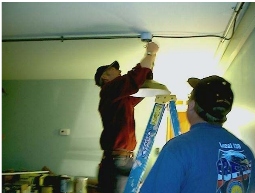
John Balch and Mike McLaughlin, members of the International Brotherhood of Electrical Workers Local 139, install the electricity at the new Habitat office.
