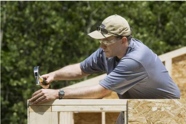
Bill Sheehy, project engineering manager at Corning Inc.'s Display Technologies division, helps tie in the walls of the Habitat house in Addison.
